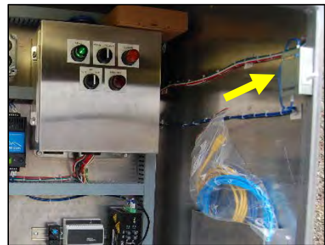
Figure 3-5. Door Alarm Switch
